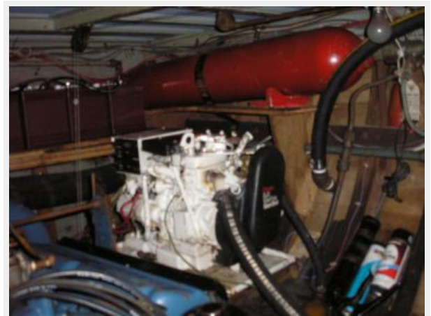
Onan Genset with Fire Suppression System
